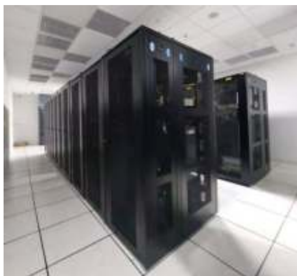
Fig 6.1 KFON ISP Room Network Rack
