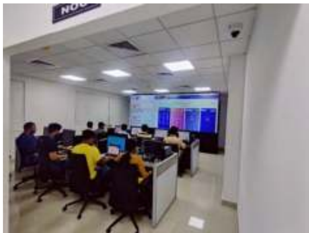
Fig 6.2 NOC Network Monitoring Room
